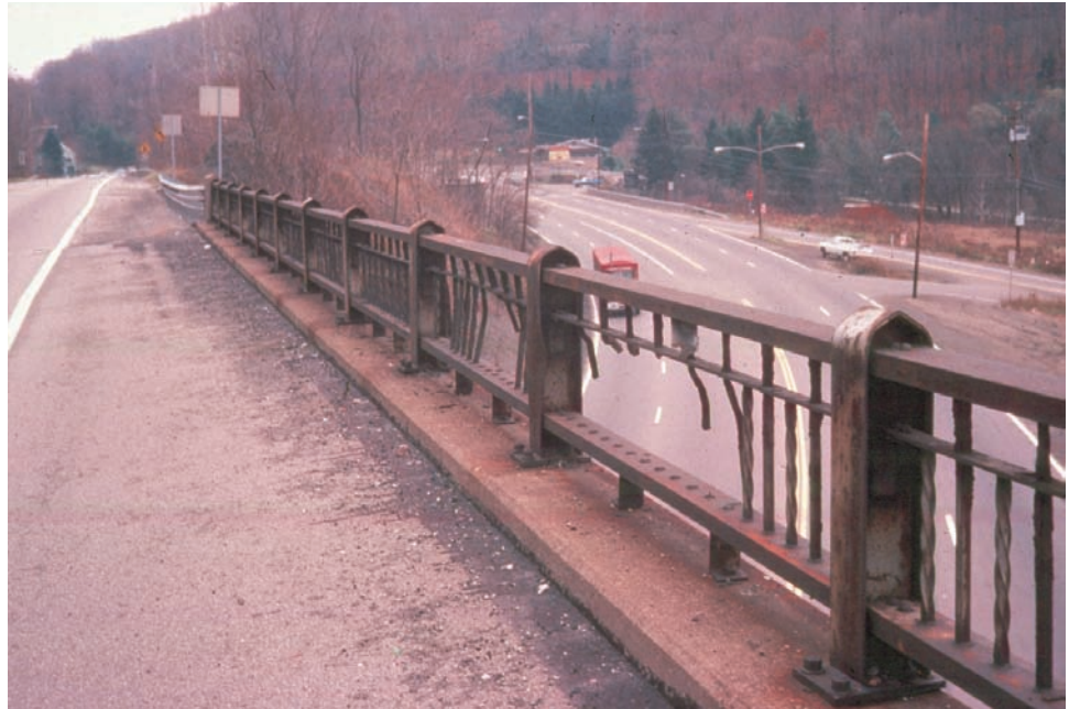
Figure 5.5.10 Damaged Steel Post Bridge Railing
