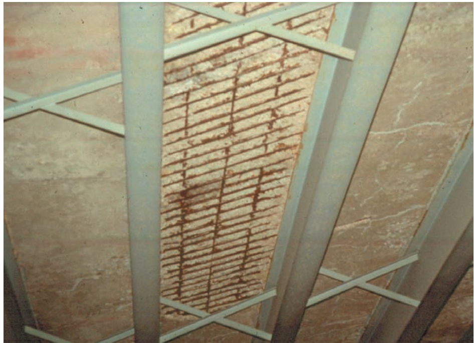
Figure 5.2.8 Spall Showing Deck Reinforcing Steel Perpendicular to Traffic
