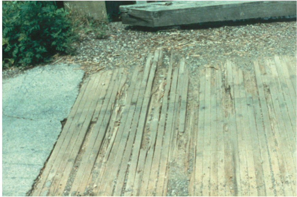
Figure 5.1.8 Wear and Weathering on a Timber Deck
