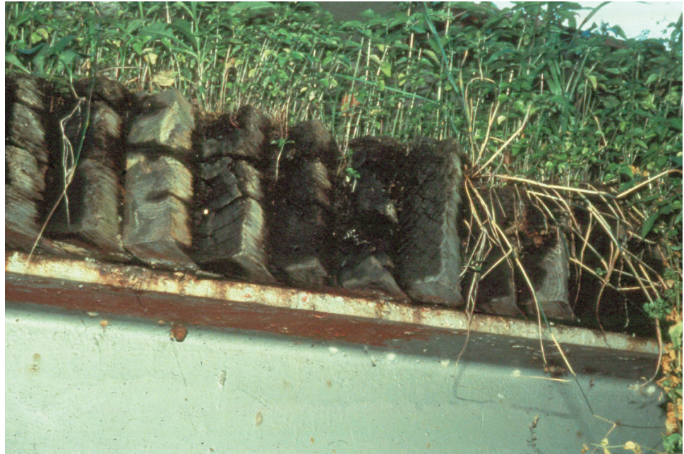
Figure 5.1.10 Edge of Deck Exposed to Drainage, Resulting in Plant Growth
