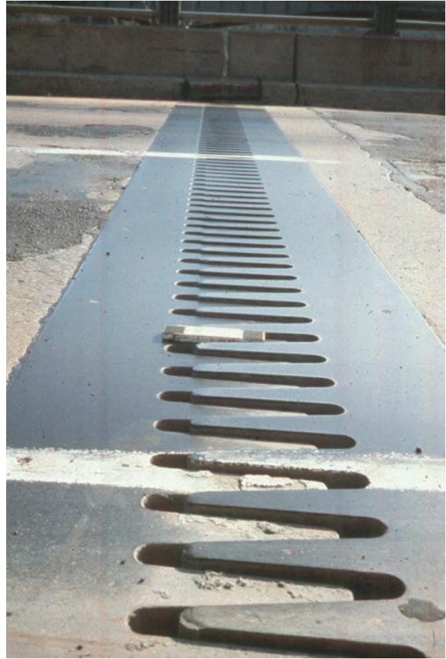
Figure 5.4.17 Improper Vertical Alignment at a Finger Plate Joint
