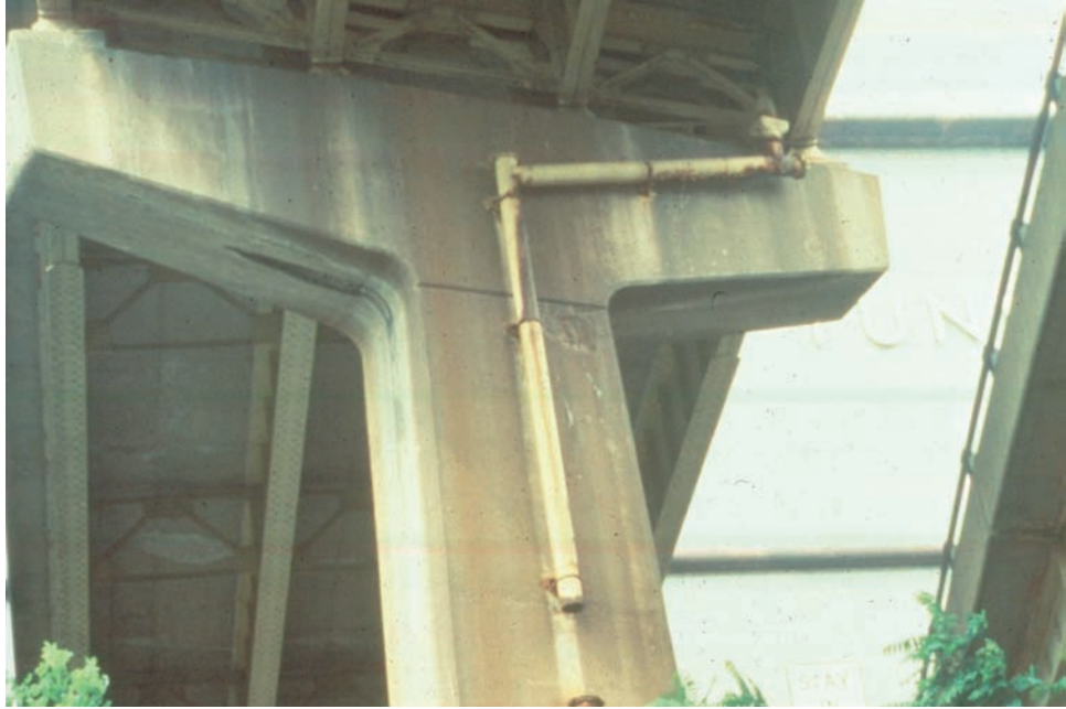
Figure 5.4.14 Downspout Pipes and Cleanout Plugs
