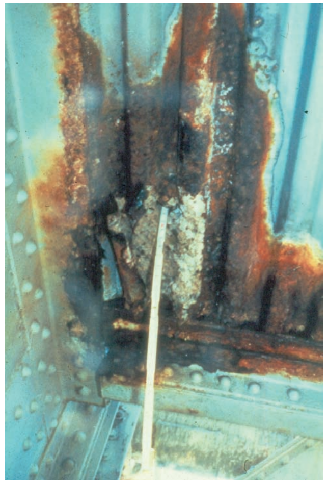
Figure 5.2.12 Deteriorated Stay-in-Place Form
