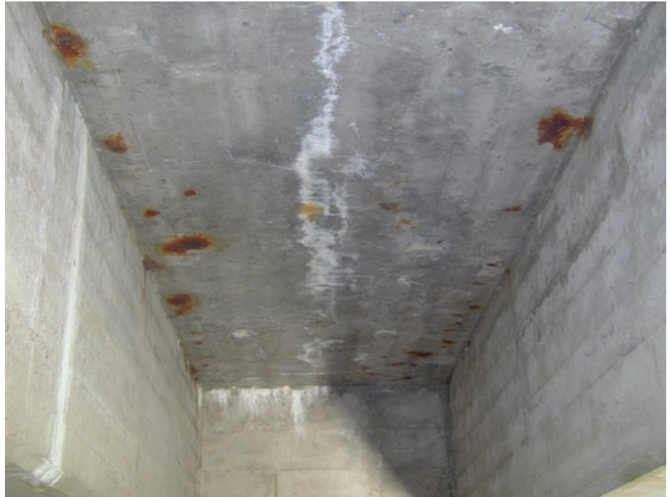
Figure 5.2.11 Underside View of Longitudinal Deck Crack
