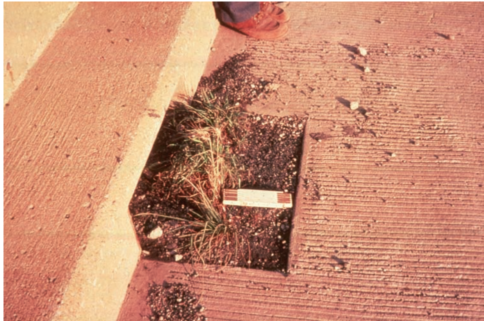
Figure 5.4.21 Clogged Drainage Inlet
